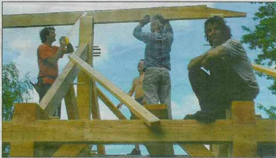
BEAM TEAM: Steve King, right, watches colleagues James Ross, left, Chris and Dave Waldon assemble the timber frame for an energy-efficient building at Fifehead Neville.
